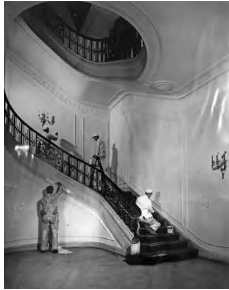
Figure 058 Entrance Hall being repainted, 1940. Evening Star , Washingtoniana Collection, DC Public Library's Special Collections.
