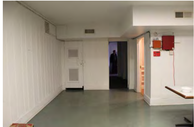
Figure 046 Typical basement floor condition. EHT Traceries.
