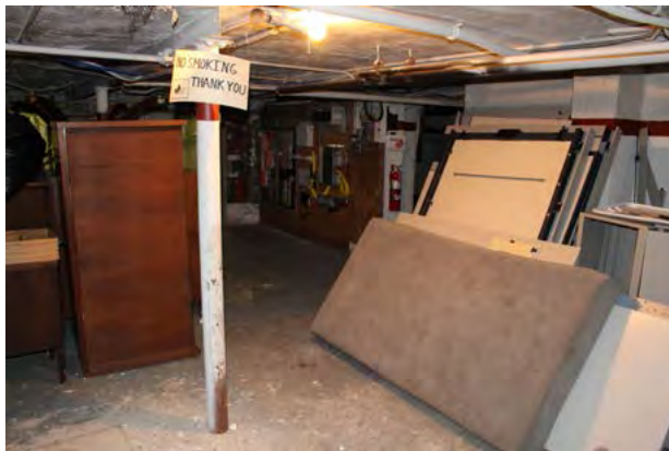
Figure 043 Typical subbasement floor condition. EHT Tracerics.
