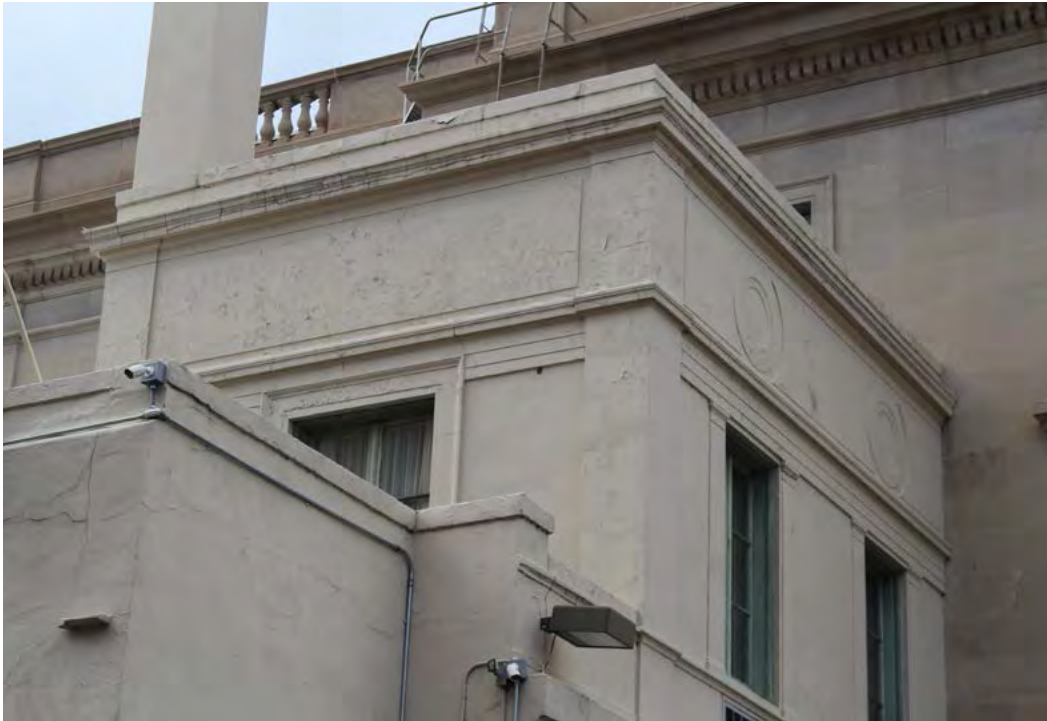
Figure 028 Detail of stucco ornament on second story of east elevation. EHT Traceries.
