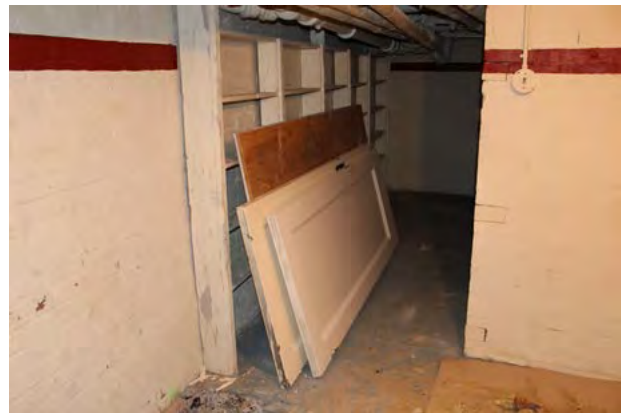
Figure 044 Typical subbasement floor condition. EHT Tracerics.
