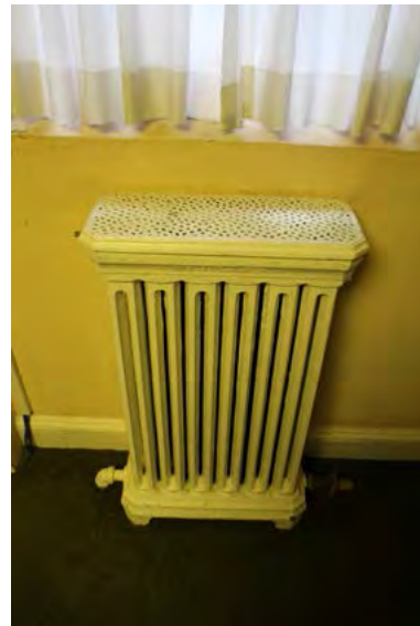
Figure 050 Original radiator (stamped 1885) on basement floor. EHT Traceries.
